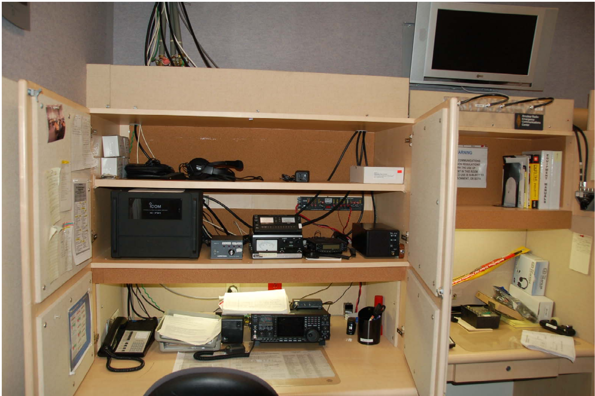
Radio Room Operating Position #1
