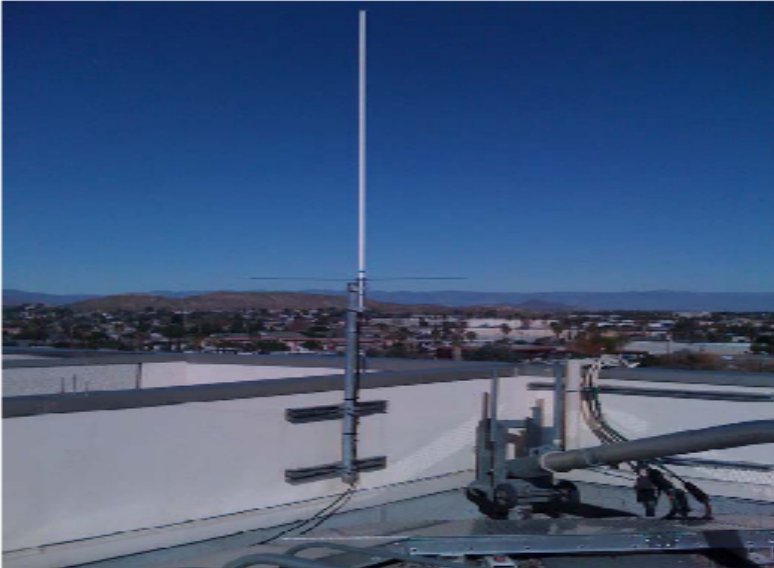
GP-15 Antenna on north end of MOB Roof
