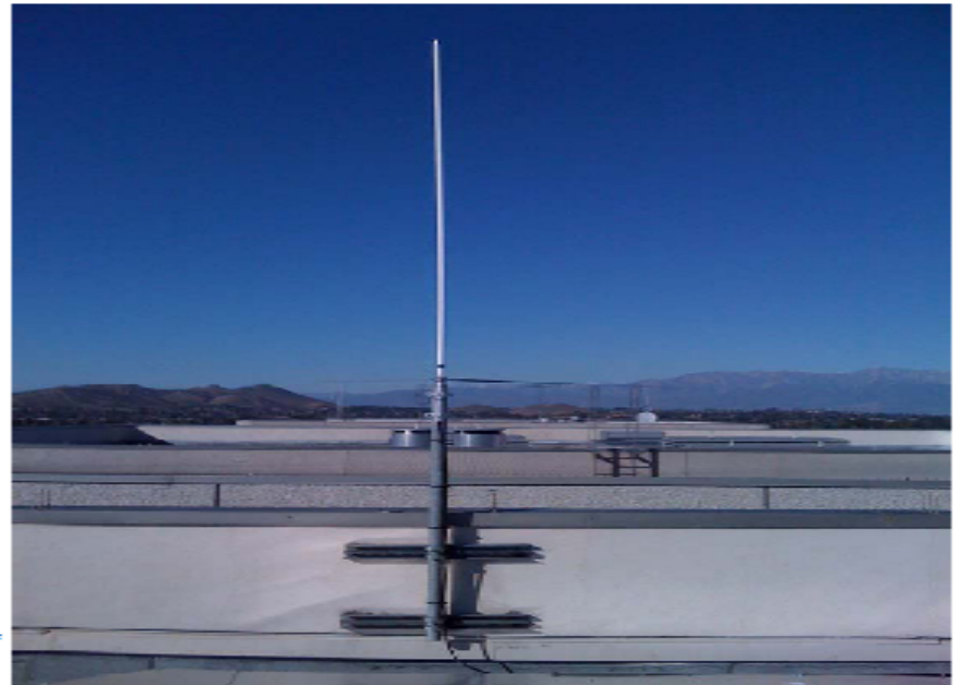
GP-15 Antenna on south end of MOB Roof
