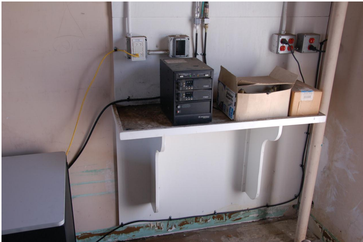
Connections to KPIT Network, Antenna, and A.C. (E-Power Outlet)
