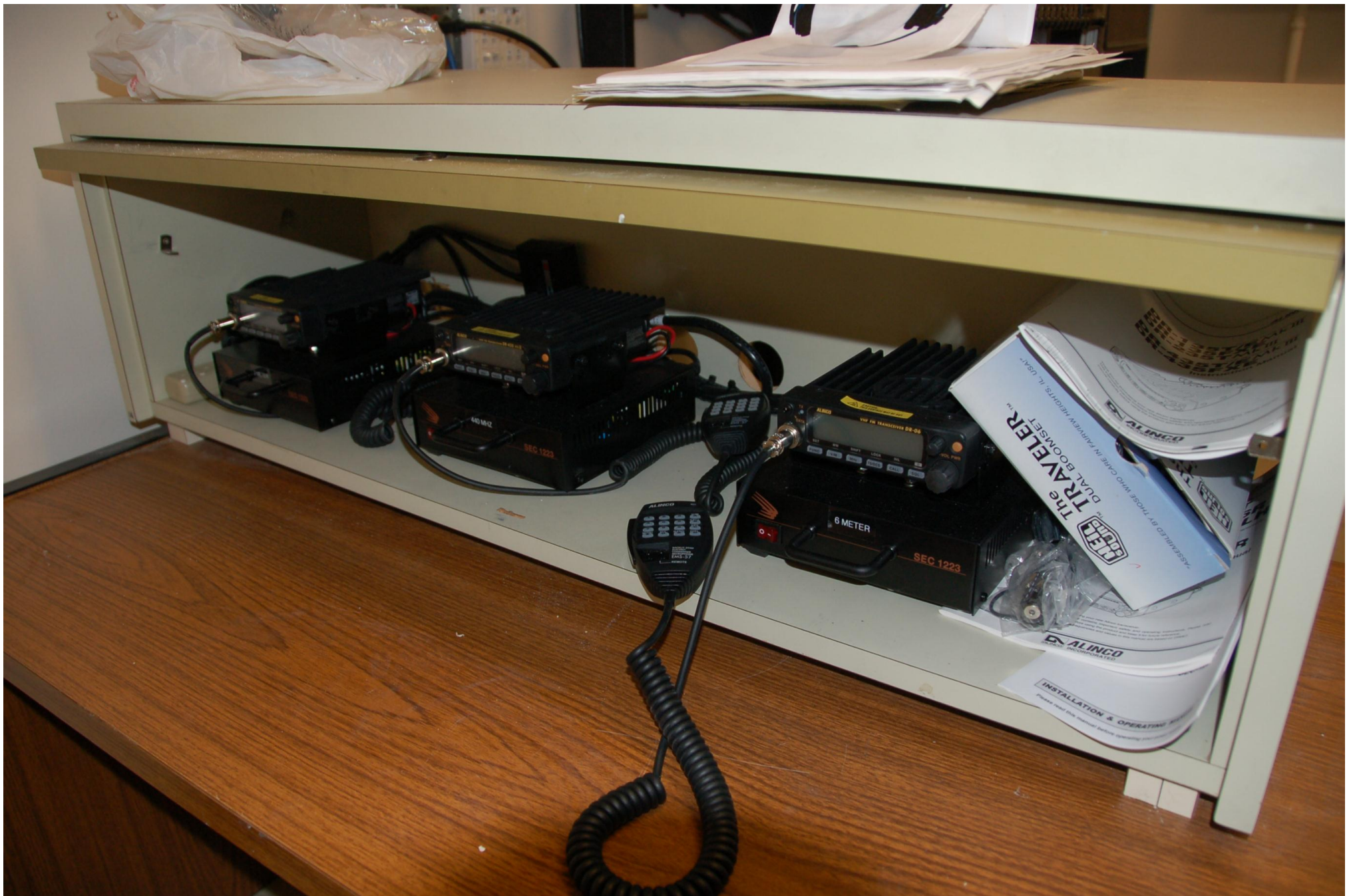
Radio Equipment in 5 th Floor “EOC”
