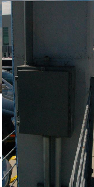
NEMA Enclosure at tower base. Houses EMP and connects to hardline runs to radios.
